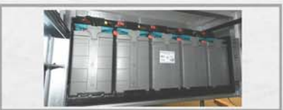
2 -> 50Kwh Energy Storage
